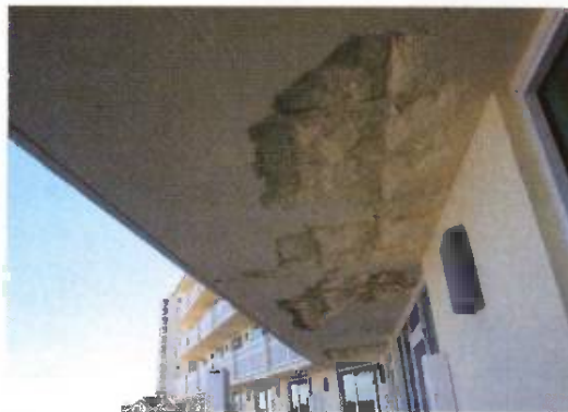
Severe underside spalling of balconies
