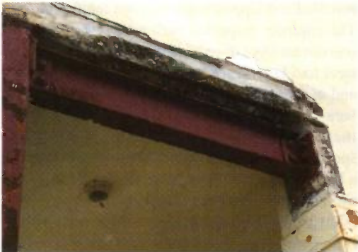
Corroded beams and columns were not capable of supporting loads much longer
