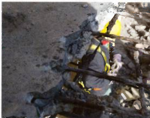
Reinforcing steel was extensively corroded
