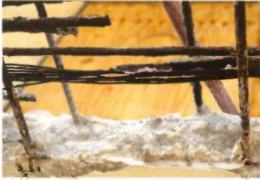
Close-up view of corroded reinforcing steel
